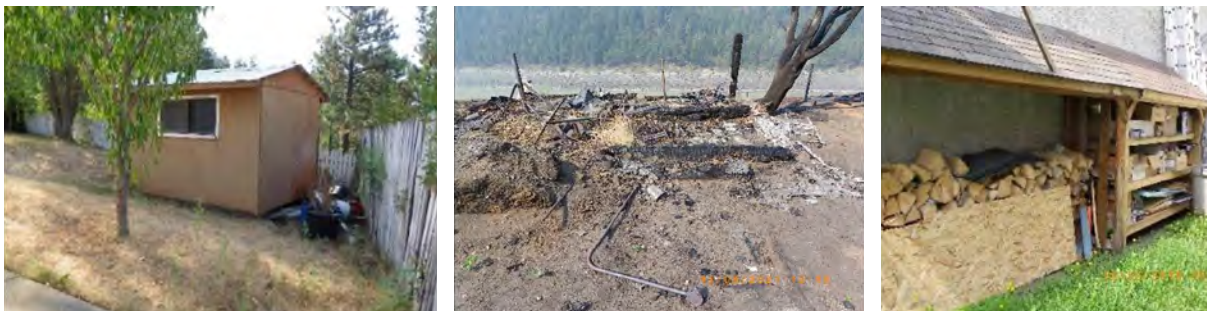
Figure 18: Outbuildings such as the shed on the left are ignition vulnerable from fire spreading in dead grass, flammable debris or a wood fence to contact and ignite it or directly ignite from burning embers such as the firewood on the right. Once ignited, the burning outbuilding or adjacent firewood ignites the house or business.
