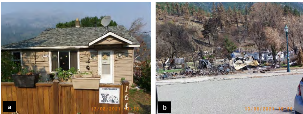
Figure 20a: Thermally softened vinyl siding on the upper third of the front facing burning structures across Fraser St. Note the wood fencing closer to the thermal source without char. Figure 20b: Burned structures across Fraser St. produced the thermal radiation that damaged the vinyl. These structures are identified in the coarse dashed yellow rectangle of Figure 17.
